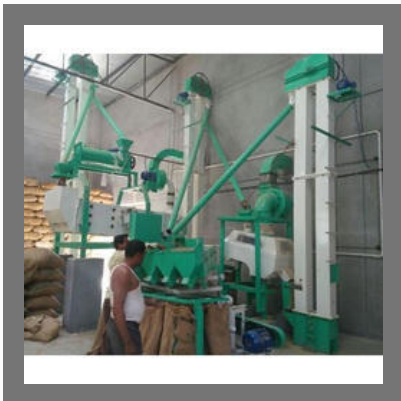
Grains Cleaning Plant
