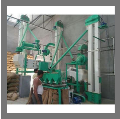
Pulses Cleaning Plant
